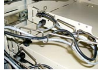
Network & AC Cabling to each Drawer
