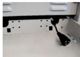
AC Cabling to each drawer
